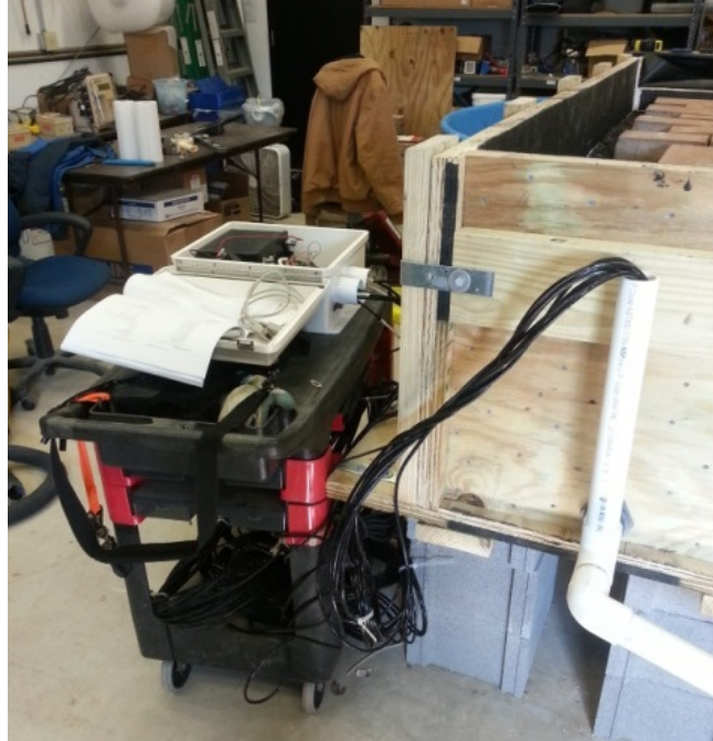
Figure 22: Instruments wired to the data logger
